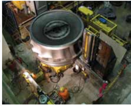
Hydro-Electric & Pumped Storage
