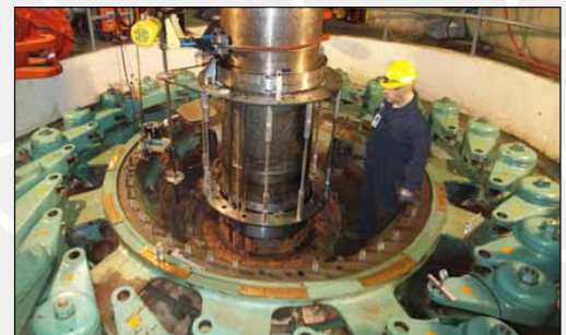
Machine Sleeve on Turbine Shaft Seal
