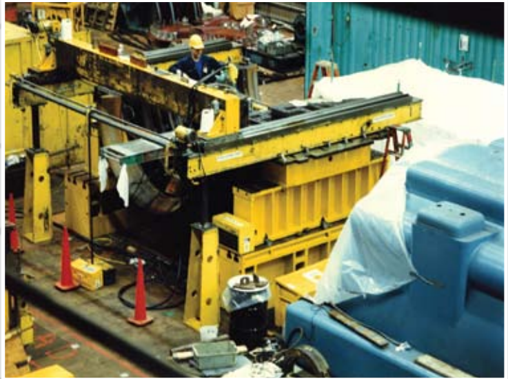
Machine Turbine Upper Case Horizontal Joint
