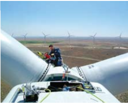
Wind Power Generation
