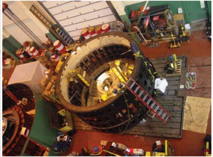
Machine Generator Stator TEE Slots
