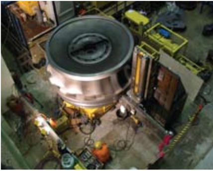
Hydro-Electric Power Generation
