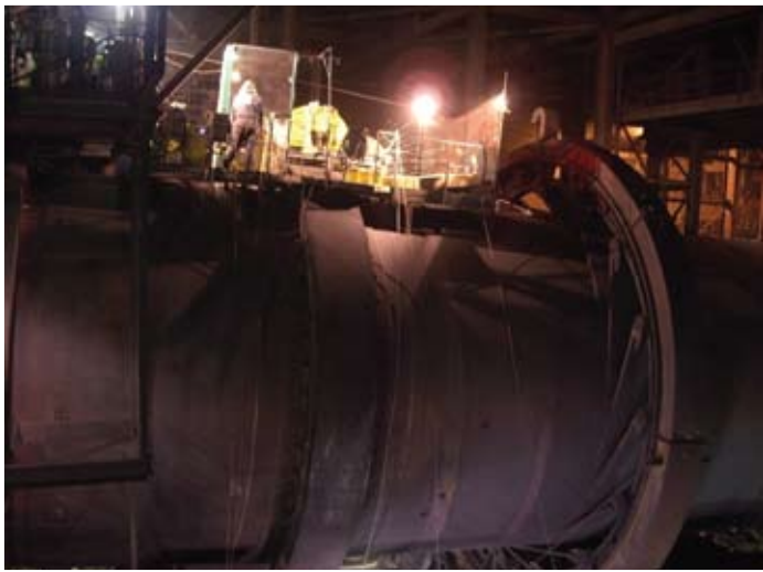
Abrasive Saw Cut Cracked Kiln Tire
