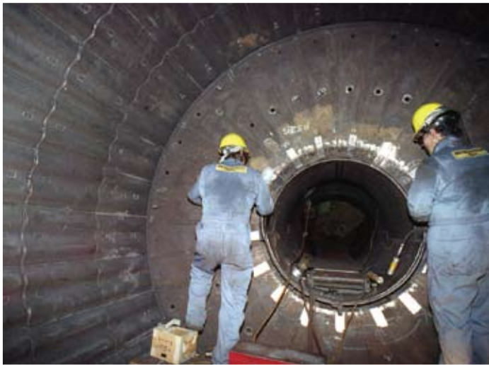
Metalstitch® Cold Cast Iron Repair of Ball Mill Head
