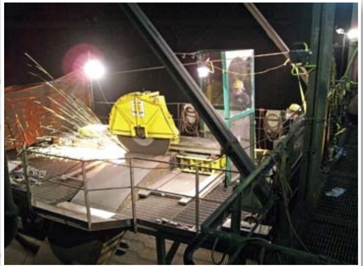
Abrasive Saw Cut Cracked Kiln Tire
