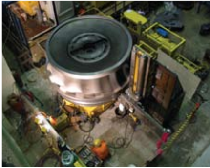
Hydro-Electric Power Generation
