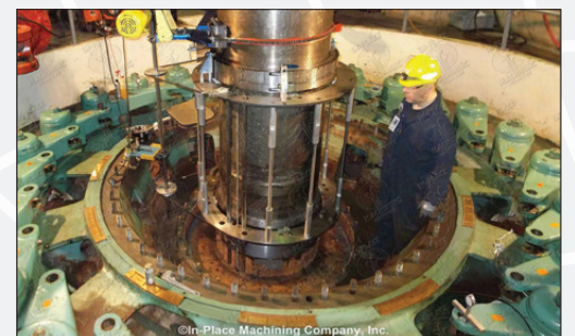
Machine Sleeve on Turbine Shaft Seal
