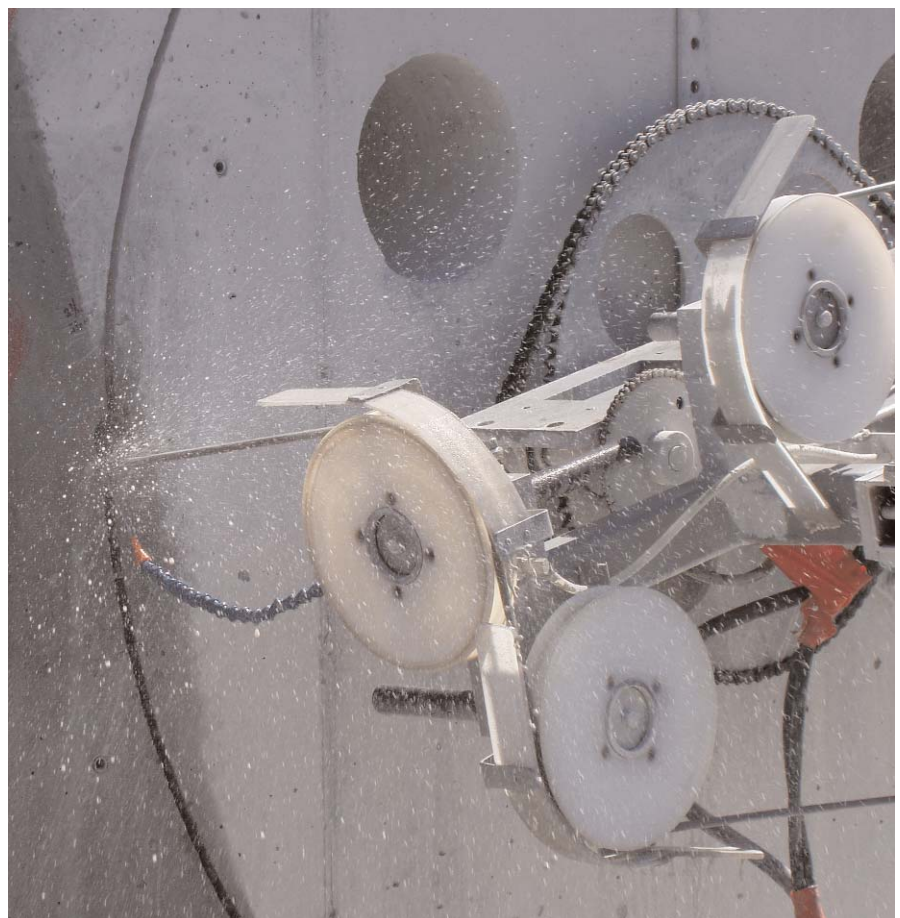
Top: Team CSDA ready to complete the 6-foot-diameter circle cut. Bottom: The wire saw completes the final cut to free the 6-foot-diameter core.
