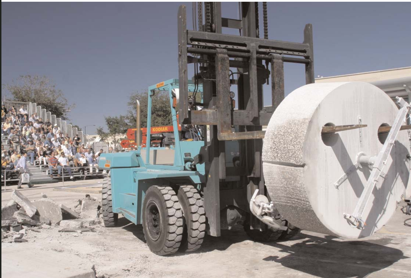
A mega concrete core is removed during a wire sawing demonstration at World of Concrete.
